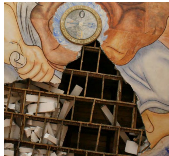
Figure 3.b.13: Damages at the dome, by seismic movement on february 27, 2010 at Chillán (picture 2010).
